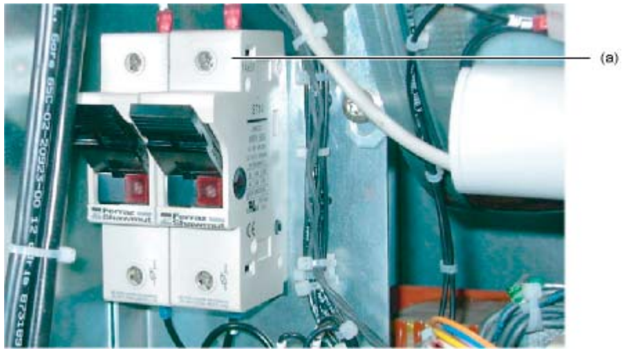
Figure 8-28 Measuring point, auxiliary power supply, fan supply bottom, frame sizes FX and GX
