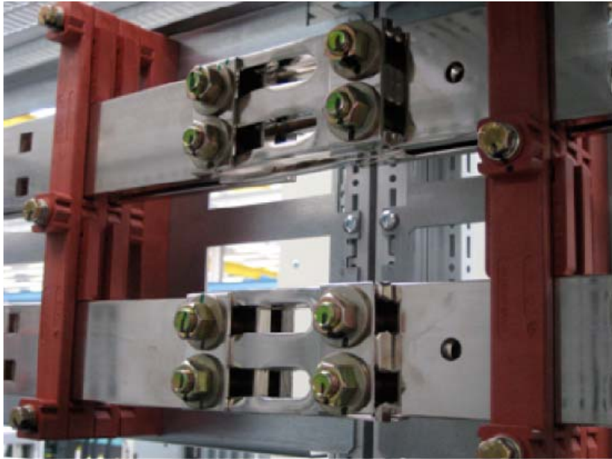
Figure 8-44 M80 to M87, DC busbar
